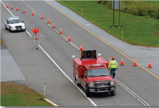
Figure 3.17 – A proper position for a flagger in the closed lane of traffic.
