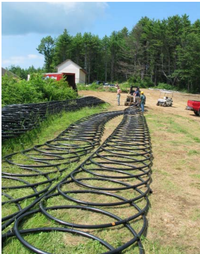
The installation of geothermal technology will reduce our dependence on fossil fuels by 65%.
