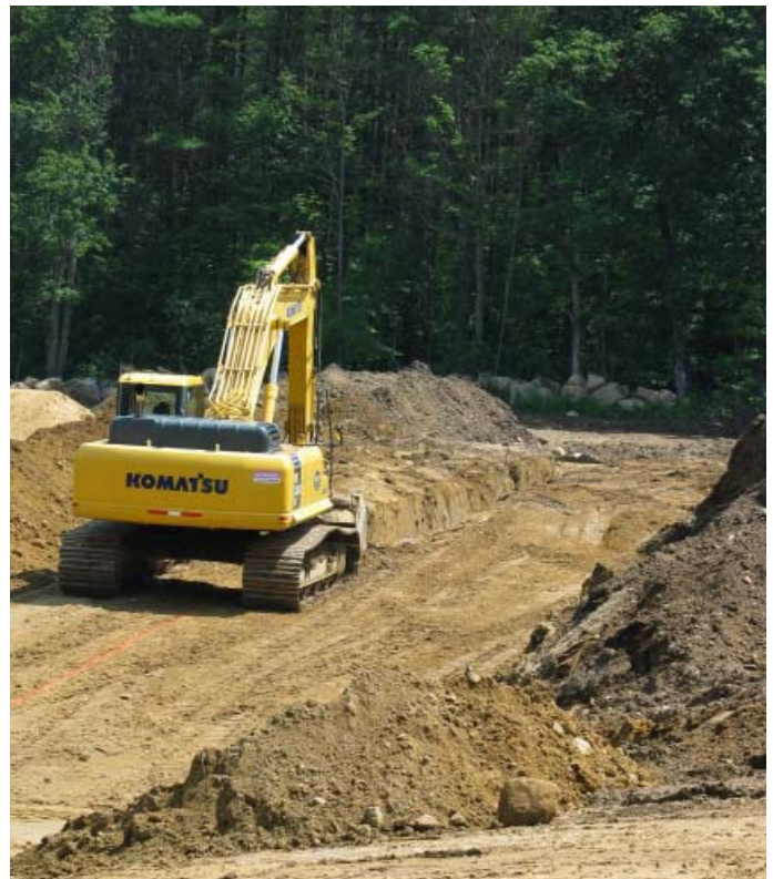
Going Green: We now have 90 geothermal wells at a depth of 310 feet, and four large horizontal well fields.
