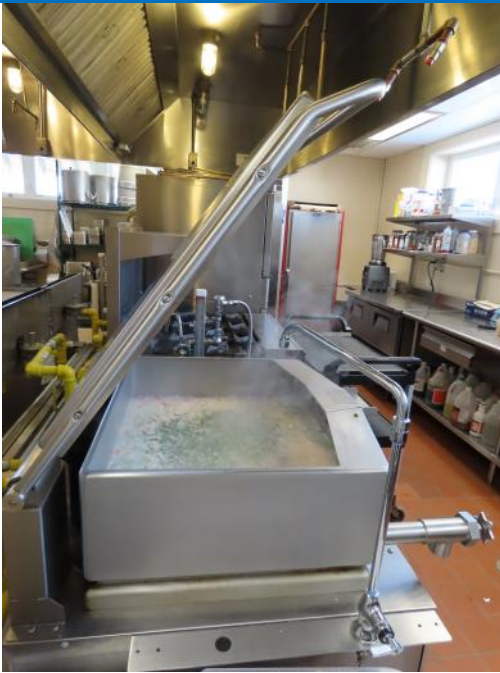
New equipment in use in the completed kitchen.
