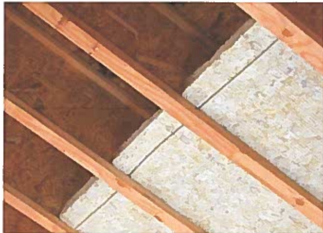
Installing mineral wool between I-joists is one of several methods builders and installing dealers can use to meet the IRC provisions.
