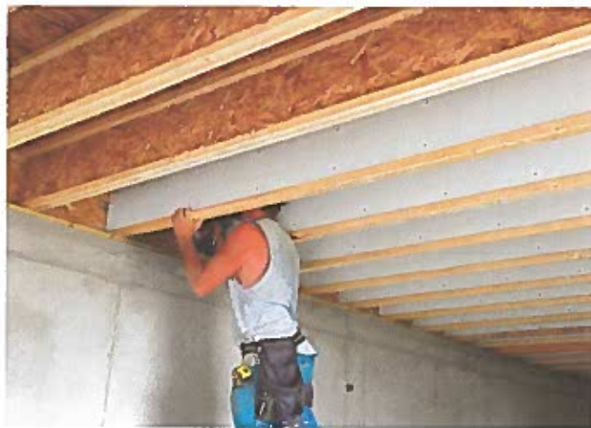
Installing 1/2-inch gypsum board to I-joist webs is one of several methods builders and installing dealers can use to meet the IRC provisions.
