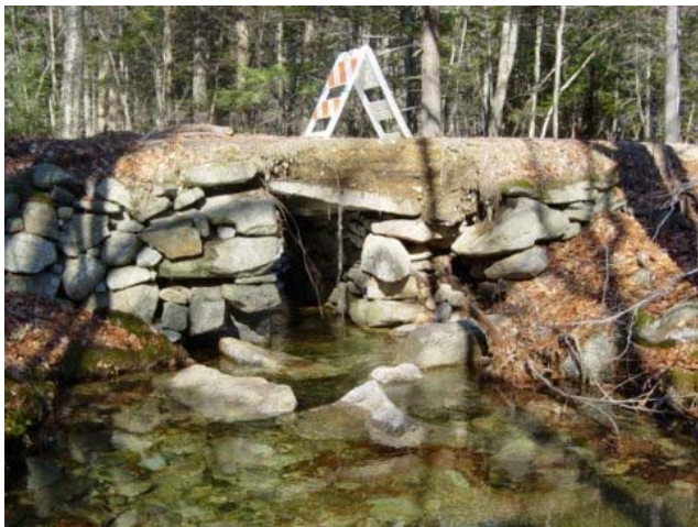
Dry-laid stone box culvert on Gore Road, Warner, NH, with minor flood damage. Photograph by James L. Garvin.
