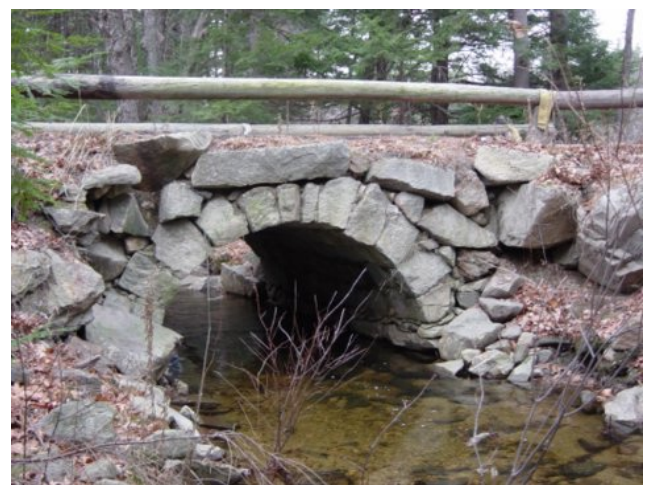
Dry-laid arched culvert, Memorial Highway over Temple Brook, Temple, NH. Photograph by James L. Garvin.
