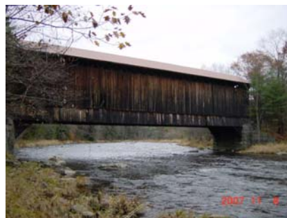
Wright's Covered Railroad Bridge (1906), Newport, N. H. (Photograph by James L. Garvin)
