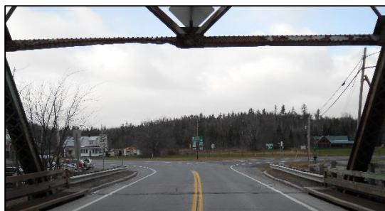
FIGURE 2 - DAMAGE TO INBOUND OVERHEAD
