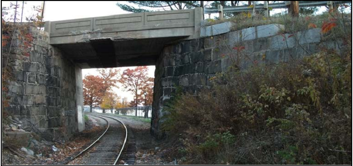
Elevation view of existing bridge, looking north along NHRR towards the Weirs
