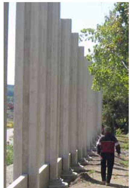
Charlie Hood checks out a sound wall construction project in September of 2009.
