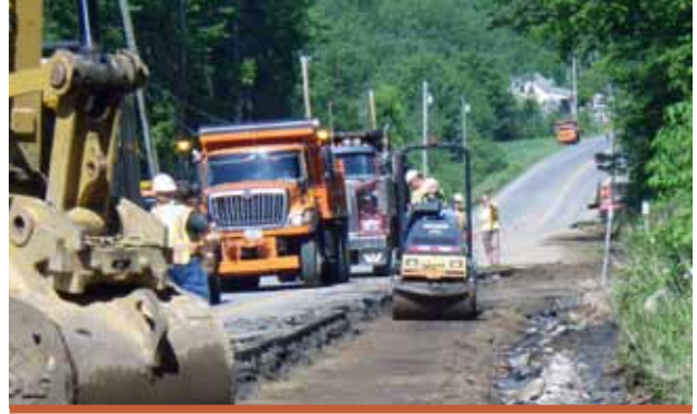
District 4 crews worked quickly to repair and reopen damaged roads in several communities.
