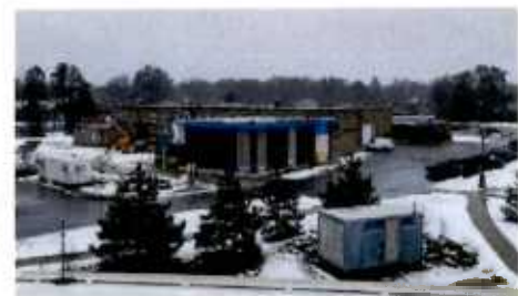
Building M undergoing a 4,574 SF addition supporting cyber readiness of the NHARNG.
