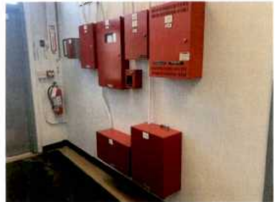
Monaco fire alarm panels protect base facilities.
