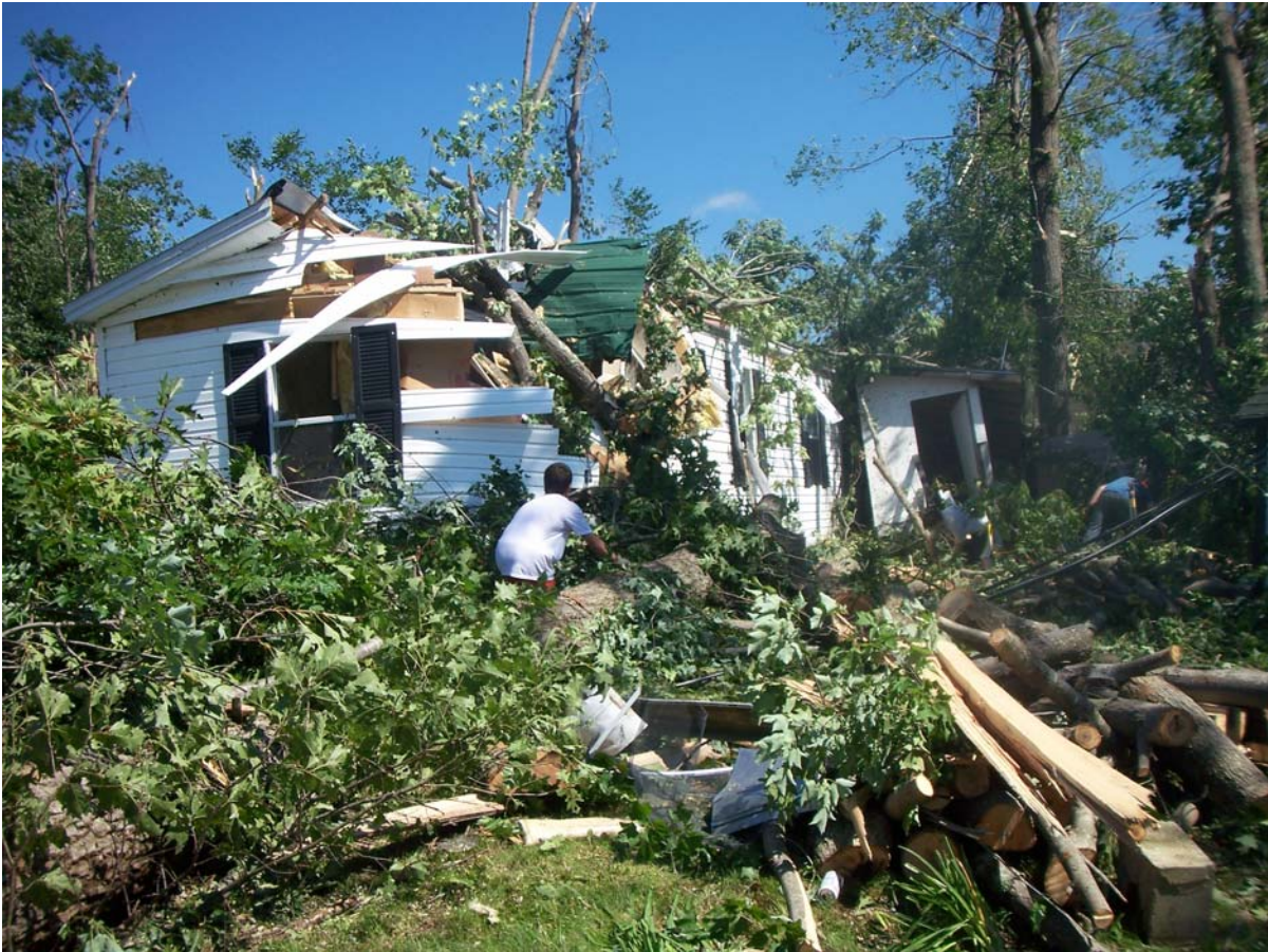
Tornado damage to a home along Northwood Lake in Epsom, one of the hardest-hit communities
