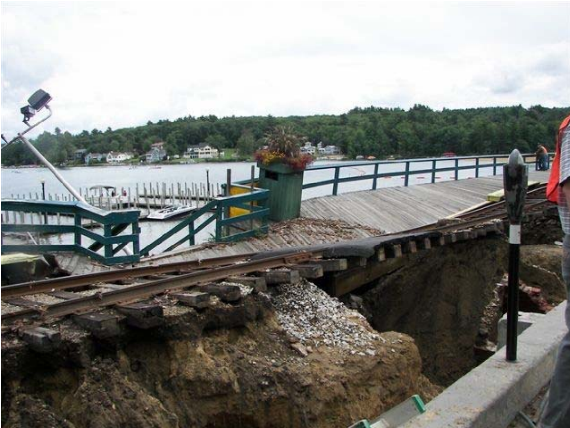
Flash flood damage to the railroad track and boardwalk at Weirs Beach. Photo by HSEM Senior Field Representative Cindy Richard.
