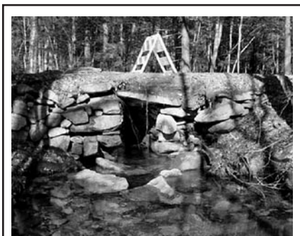
Dry-laid stone box culvert on Gore Road, Warner, NH, with minor flooding damage. Photograph by James L. Garvin
