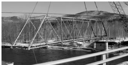
The northeast span of the Meadow Bridge in Shelburne (1897) is lifted by crane from the shore of the Androscoggin River, February 25, 2004. Photograph by Ray Danforth.
