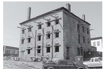
South elevation of the Eagle Block, showing work in progress. (Photograph by James L. Garvin)
