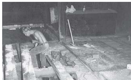
At work on the foundation of the Josiah Bartlett Barn in Kingston. A horse shed was later added to the rear of the structure. (Photograph by Elizabeth H. Muzzey)
